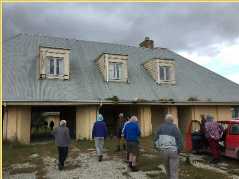
Abandoned about a decade ago, the once-magnificent mansion is now in a state of considerable disrepair – CFE
